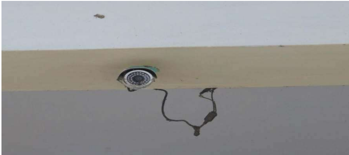
(SOME OF THE CCTV CAMERAS INSTALLED AT VARIOUS LOCATIONS IN THE CAMPUS)
